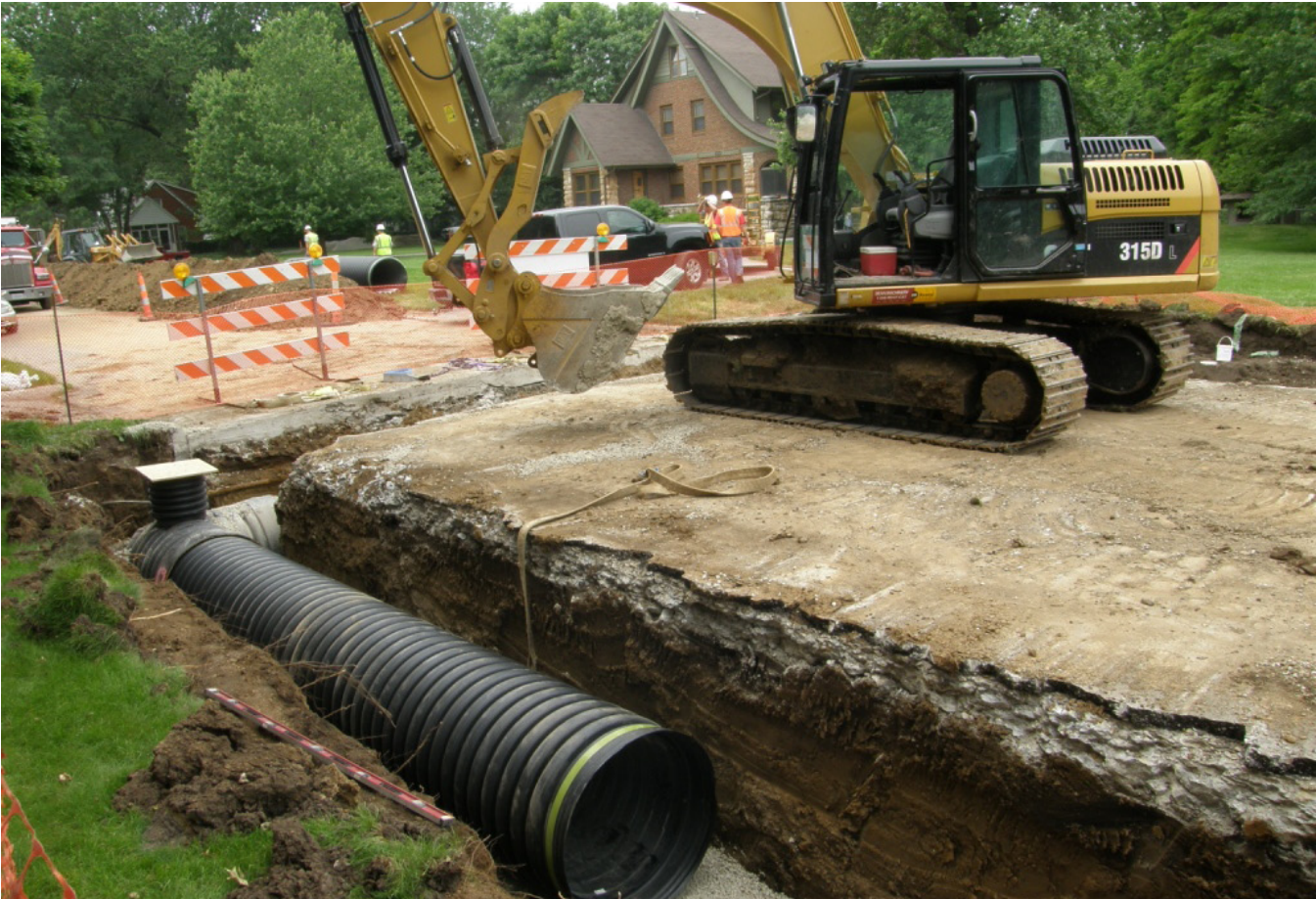
Bioretention cell below-grade storage, Middle Blue River Basin Green Infrastructure Pilot Project
