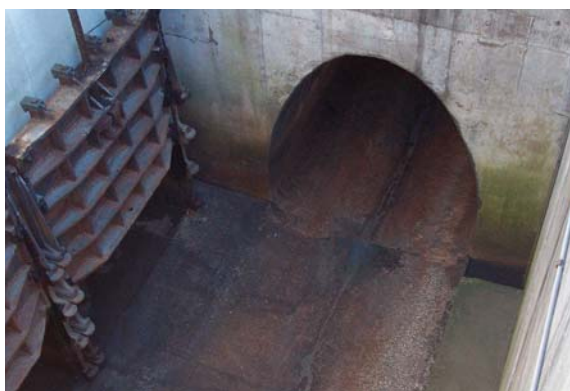
Diversion Structure - Blue River WWTP
